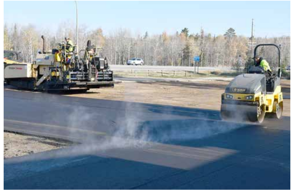
LOOKING GOOD— Construction crews have been busy repaving the parking lot at the Y Store. The project will be finished by Friday, November 4th.
